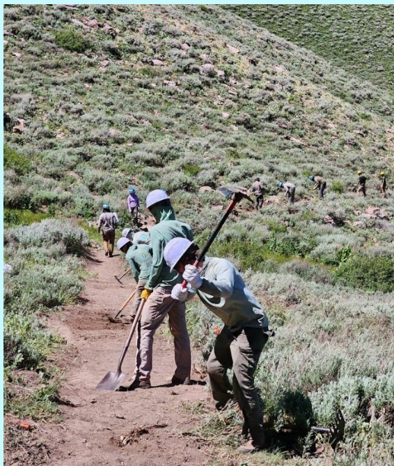
New tread on the Stansbury Crest Trail with the SLRD Trails and Wilderness Crew. Photo credit: David Wyllie
