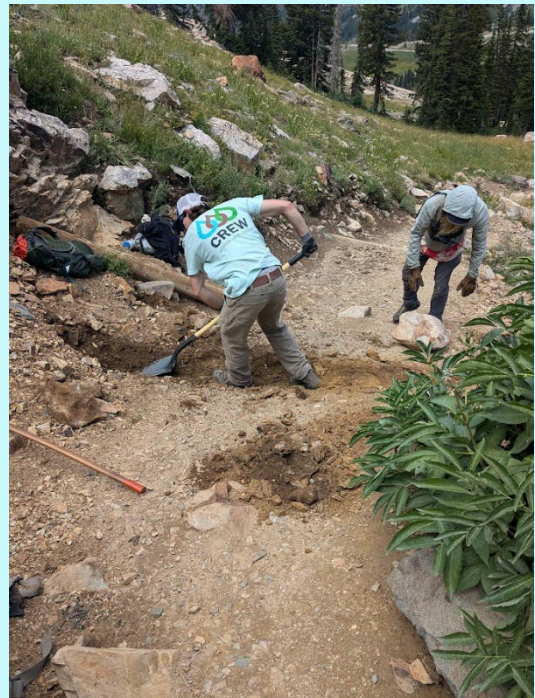
Rebuilding check steps with the Alta Environmental Center crew on Cecret Lake Trail. Photo credit: Emily Salle
