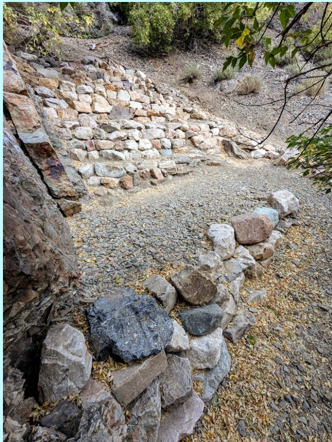
Partial view of the finished product after 11 weeks of work. Photo credit: Emily Salle
